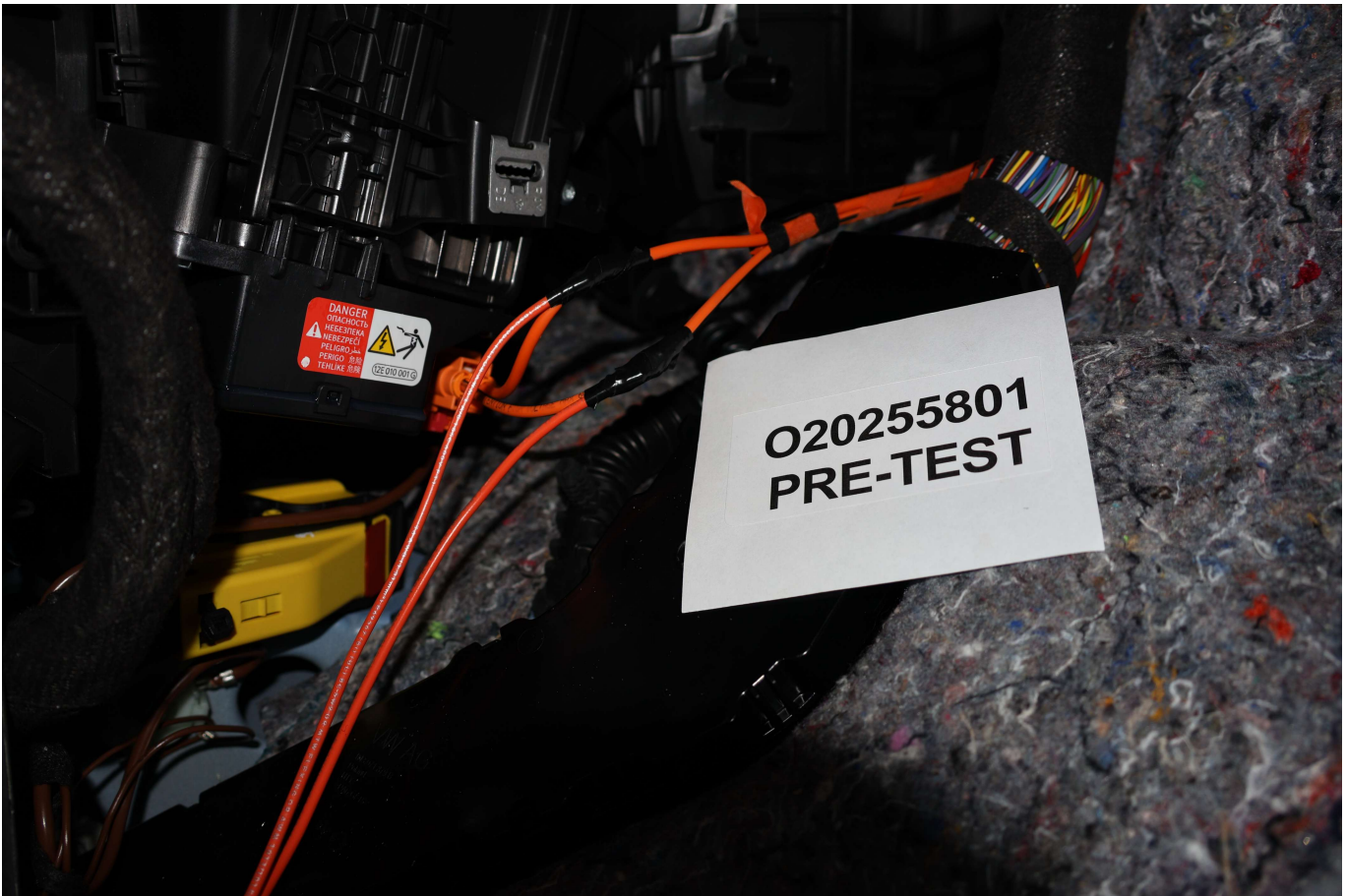
Photo No. 305-22 - Pre-Impact View of High Voltage Leads Attached
